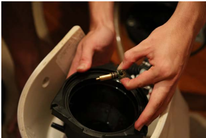
Its out! NOTE: the two O-rings. *IMPORTANT* Loss of system pressure without losing bowl water can occur at this junction
